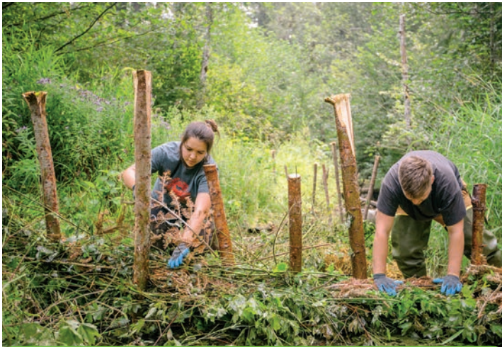
3 Workers pile up debris and pound stakes into the stream in areas where beavers will be released. That can encourage beavers to build dams there.
